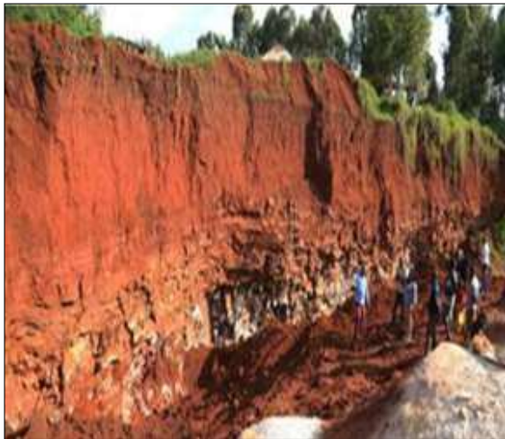
C. Loose Topsoil and Soapstone Rocks
