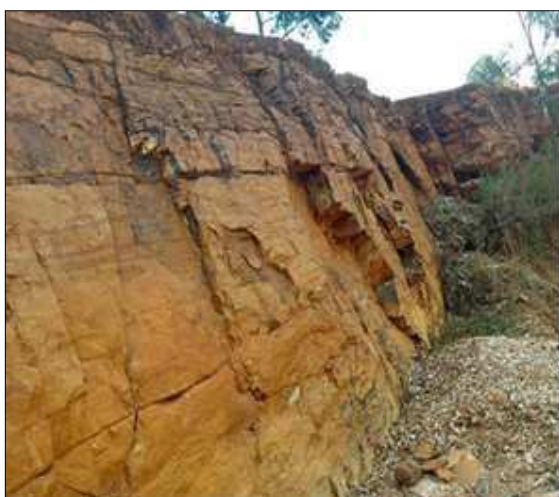
A. Rock Discontinuities (joints, cracks)
