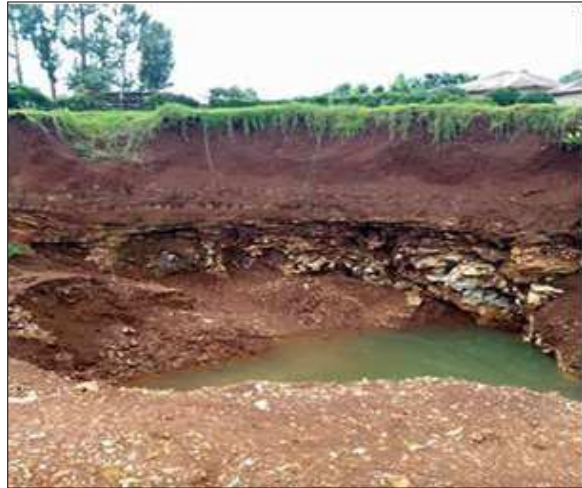
D. Water Infiltration through Slope Face
