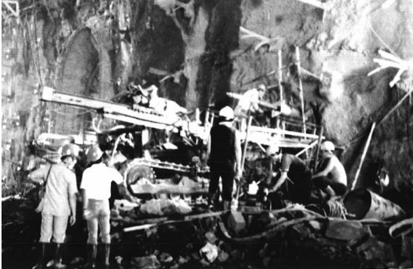
Figure 11.21: Installation of cables in the sidewall of the power cavern of the Mingtan project in Taiwan.
