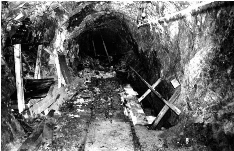
Figure 11.3: An accumulation of small blocks and wedges which have fallen from the roof and walls of an unsupported tunnel in a closely jointed rock mass. These small failures, induced by mining activities in adjacent stopes, could be controlled by the installation of light support systems such as those illustrated in Figures 11.1 and 11.2. A layer of shotcrete can provide very effective support for this type of rock mass.
