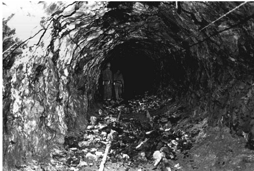
Figure 6.5: Ravelling of small wedges in a closely jointed rock mass. Shotcrete can provide very effective support for such rock masses.
