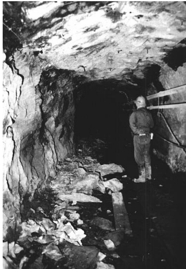
Figure 10.2: Spalling of one wall of a drive in quartzite at a depth of about 1,500 m in a uranium mine. In this case, an open stope on the left of the picture caused the stresses in the left-hand wall of the drift to be high enough to initiate spalling. This spalling is relatively minor and is parallel to the drift wall.
