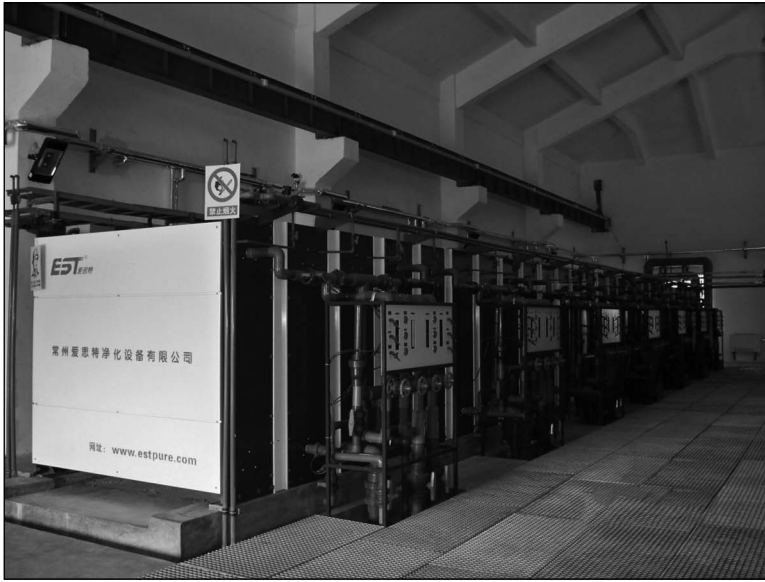
Figure 4. Yanzhou coal mine water desalination plant
